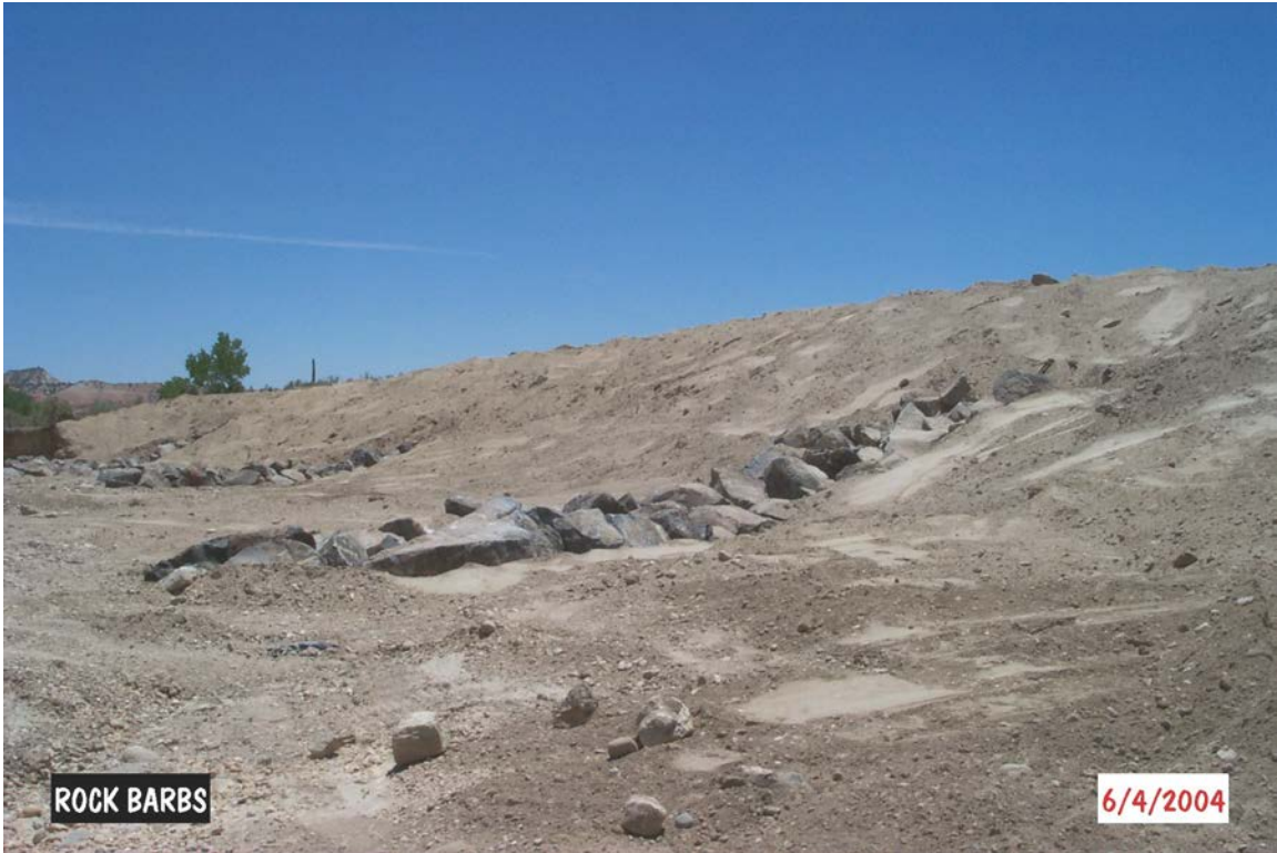
View of rock barbs and sloping on Paria River Restoration Demonstration Project, looking south from Highway 12 at Cannonville Bridge. (June 2004)
