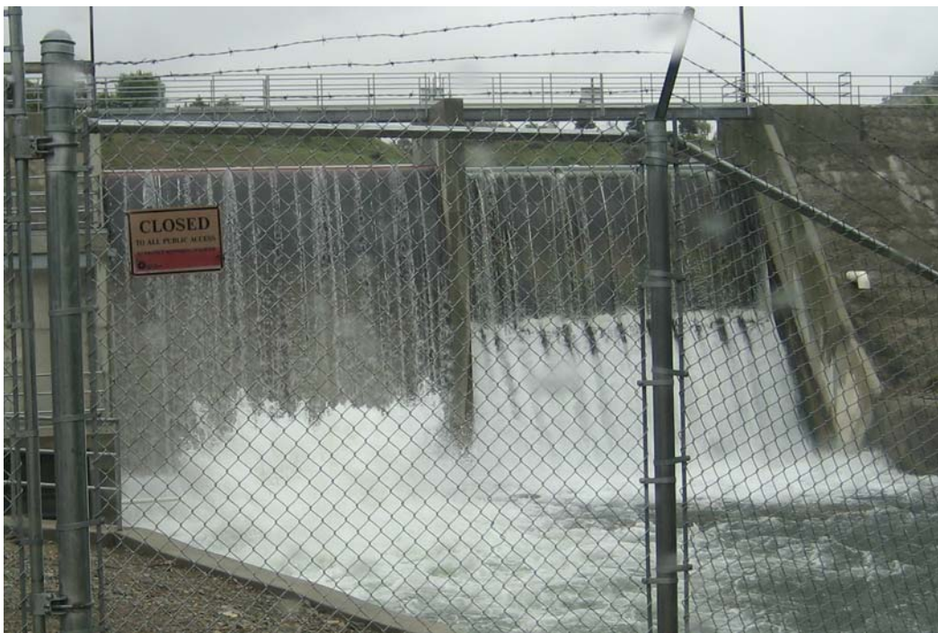
Figure 6: Use of Spillway Releases to Aerate Discharge from the Low-Level Outlets on First Dam (shown on the spillway on the left)
