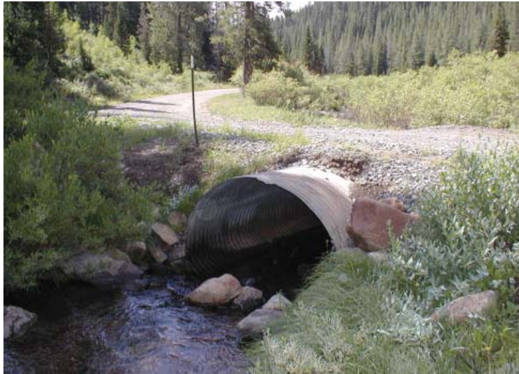
A properly sized and placed culvert will handle 50 year flood events and allow safe fish passage.
