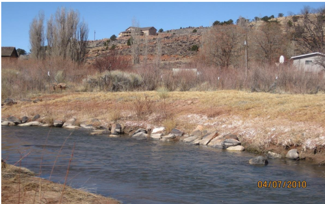
Figure 2: After: Practices installed included bank shaping, rock rip rap, rock barbs and willow planting.
